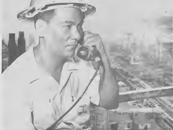
HIGH ON the 17th level of the cat cracker, J. R. Sism makes his report to the operator over a special sound power phone.
